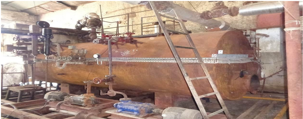
Photo 2: Boiler in bare conditions.
