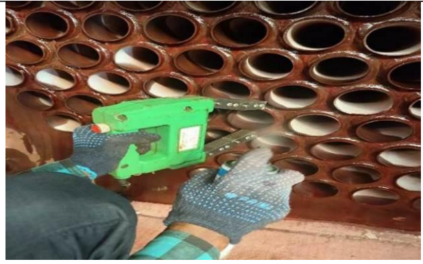
Photo 6: No surface / sub surface indication observed in Circumference & Longitudinal weld joints of steam drum in Magnetic Particle Inspection (MPI).
