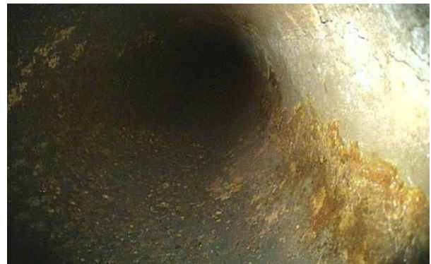
Photo 4: Minor corrosion & Scaling observed inside furnace tubes in Videoscopy inspection. It is required to clean the tubes for good operation of boiler.
