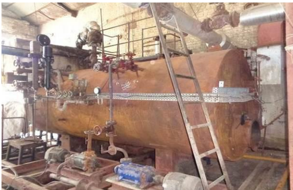
Photo 3: Externally surface shows minor corrosion, scaling. No cracks observed visually in fillet weld as well as long seams & circumferential seams weld.
