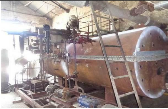
Photo 5: No surface indication observed in Circumference & Longitudinal weld joints of steam drum in Liquid Penetration Testing (LPT).
