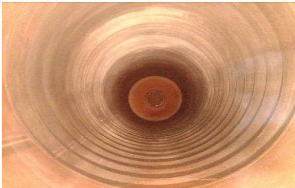
Photo 10: Internally surface shows minor corrosion & scaling. All weld joints are observed in good condition.
